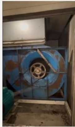
Picture 3 Water Presence Client 2
