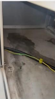
Picture 1 Water Presence Client 1
