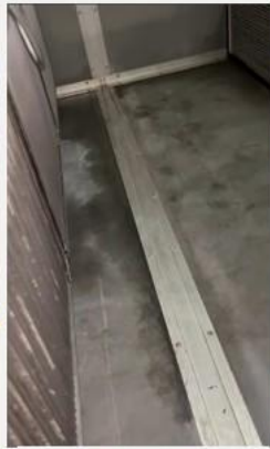
Picture 2 Water Presence Client 1
