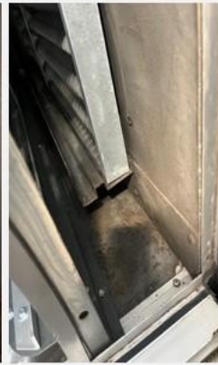
Picture 6 Filter not properly sealed Client 1
