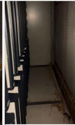
Picture 5 Water Presence Client 2
