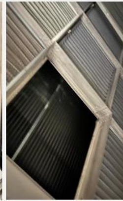
Picture 7 Only pre-filter installed – no filter Client 2
