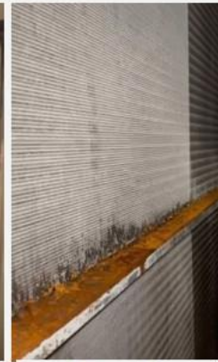
Picture 4 Water Presence Client 2
