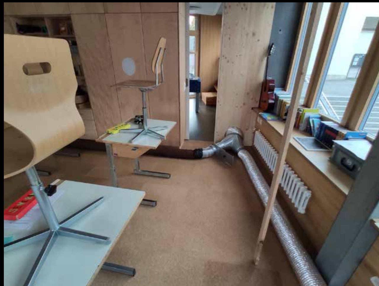
Flow recirculation by fabric-tubes
